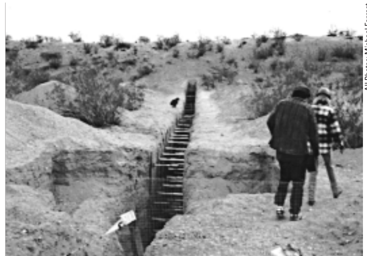
With coarse, dry gravels and sediments, sheets of plywood are unnecessary to hold back the trench walls.
