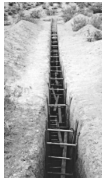
Paleoseismology is not for the claustrophobic. Dry sediments are easier to shore and offer greater peace of mind than wet ones. The Garlock trench provided a good workout for those who climbed, ducked, and crawled from one end to the other.
